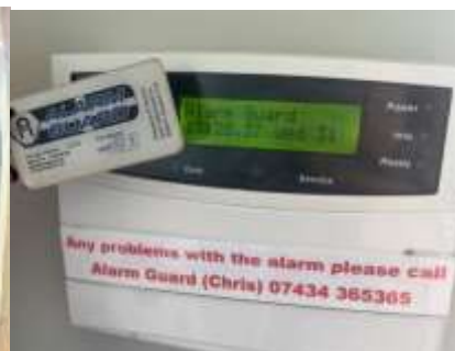
Alarm panel and fob
